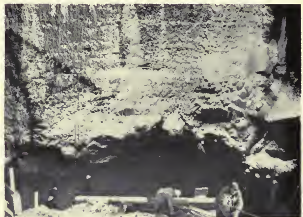
BLACK CANYON'S "STUBBED TOE." —This shows how the toe of the dam was eroded and undercut. After the cavity was cleaned out, a formation of hard, well-cemented conglomerate and sandstone was exposed, providing a firm foundation for repair.
